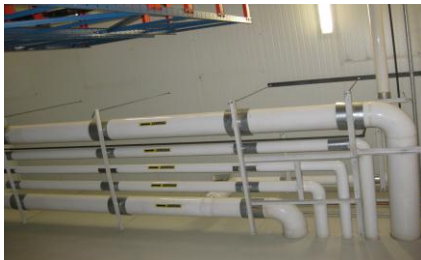
CHILLED WATER INSULATED PIPES WITH PVC CLADDING
