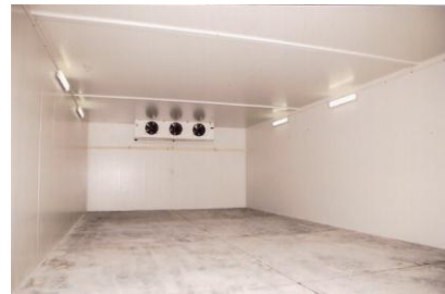
REFRIGERATION LIGHTING SYSTEM
