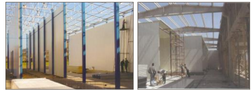
Multi Chambered Cold Stores
