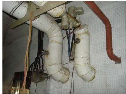
Chilled Water Pipe Insulation
