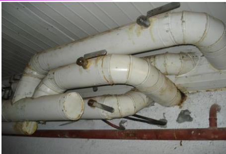
Chilled Water Pipe Insulation
