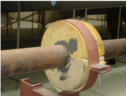
Chilled Water Pipe Support
