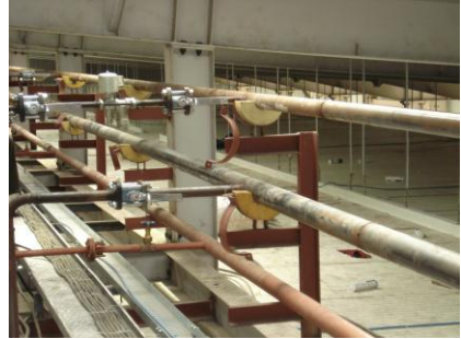
Chilled Water Piping
