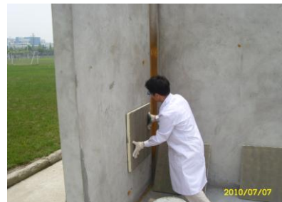
WALL INSULATION WITH PUF / PIR SLABS FIXING OF SLAB ON TO THE WALL
